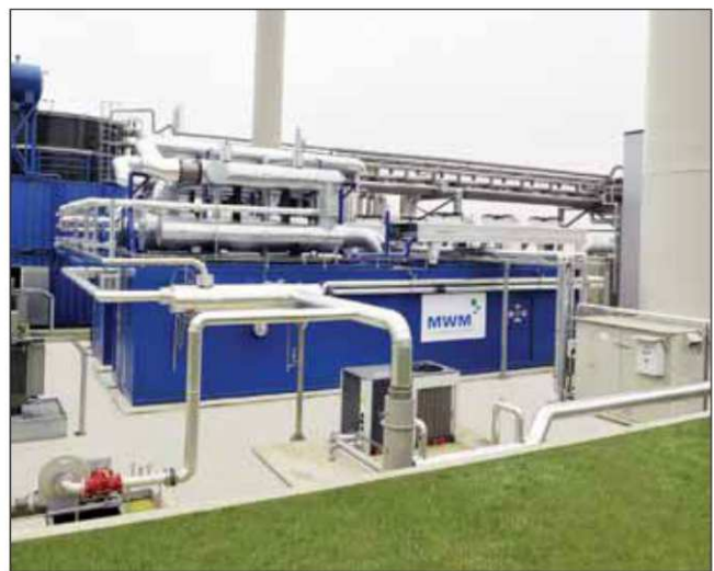
Typical CHP Installation
